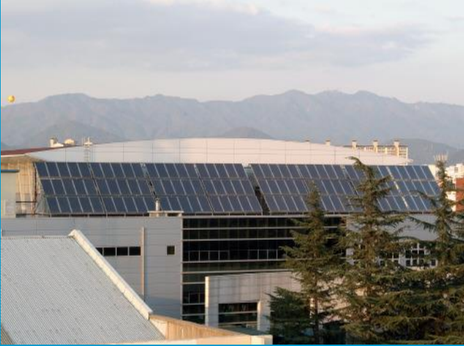
KNU Solar Thermal System, no. 120
